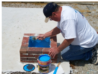
Brush or roll 2 coats of waterproofing membrane onto area to be waterproofed.
