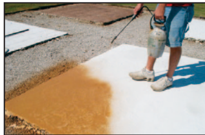
APPLY MULTI-STAIN VIA PUMP UP SPRAYER, ALLOW TO DRY, THEN ROLL ON CLEAR SEAL TO PROTECT THE FINISH.
