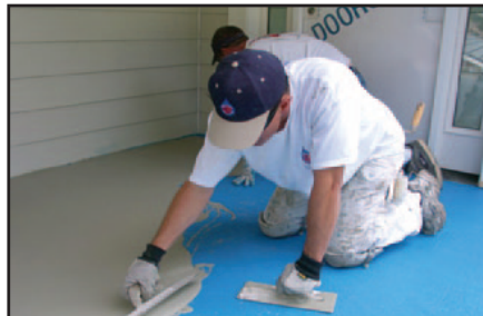
DEPENDING UPON SCOPE OF THE JOB, SCRATCH KOTE 2000 IS TROWELED OR ROLLED OVER MULASTICOAT, COVERING COMPLETELY.
