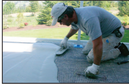
ON PLYWOOD: TROWEL MULTI-BASE INTO METAL LATHE. NO LATHE IS USED OVER CONCRETE SUBSTRATE.
