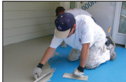
DEPENDING UPON SCOPE OF THE JOB, SCRATCH KOTE 2000 IS TROWELED OR ROLLED OVER MULASTICOAT, COVERING COMPLETELY.
