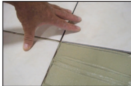
INSTALL WEARING SURFACE. PLACING OF TILE IS BEING DEPICTED. OTHER WEARING SURFACES MAY BE USED SUCH AS: STONE, BRICK, PAVERS, CONCRETE, ETC.
