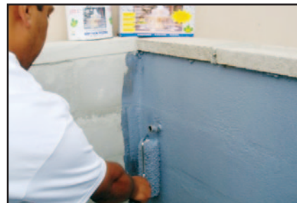
ROLL OR BRUSH WATERPROOFING MEMBRANE ON THE REMAINING SURFACES TO BE WATERPROOFED
